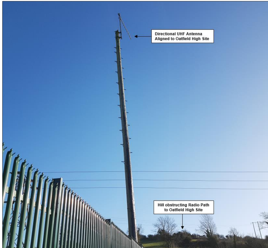
Figure 9. UHF Antenna at Tulla 38 kV site (aligned into hillside).
