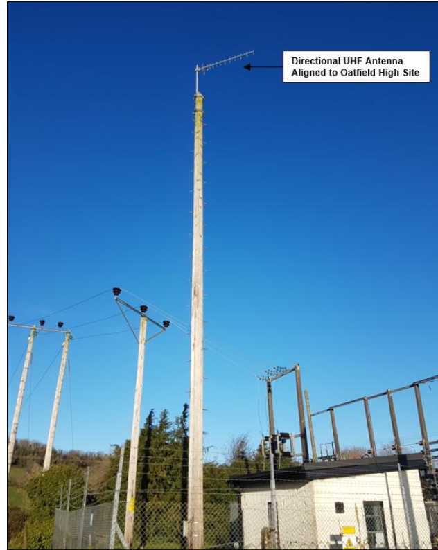
Figure 26. UHF Antenna at Drumquin 38 kV site.
