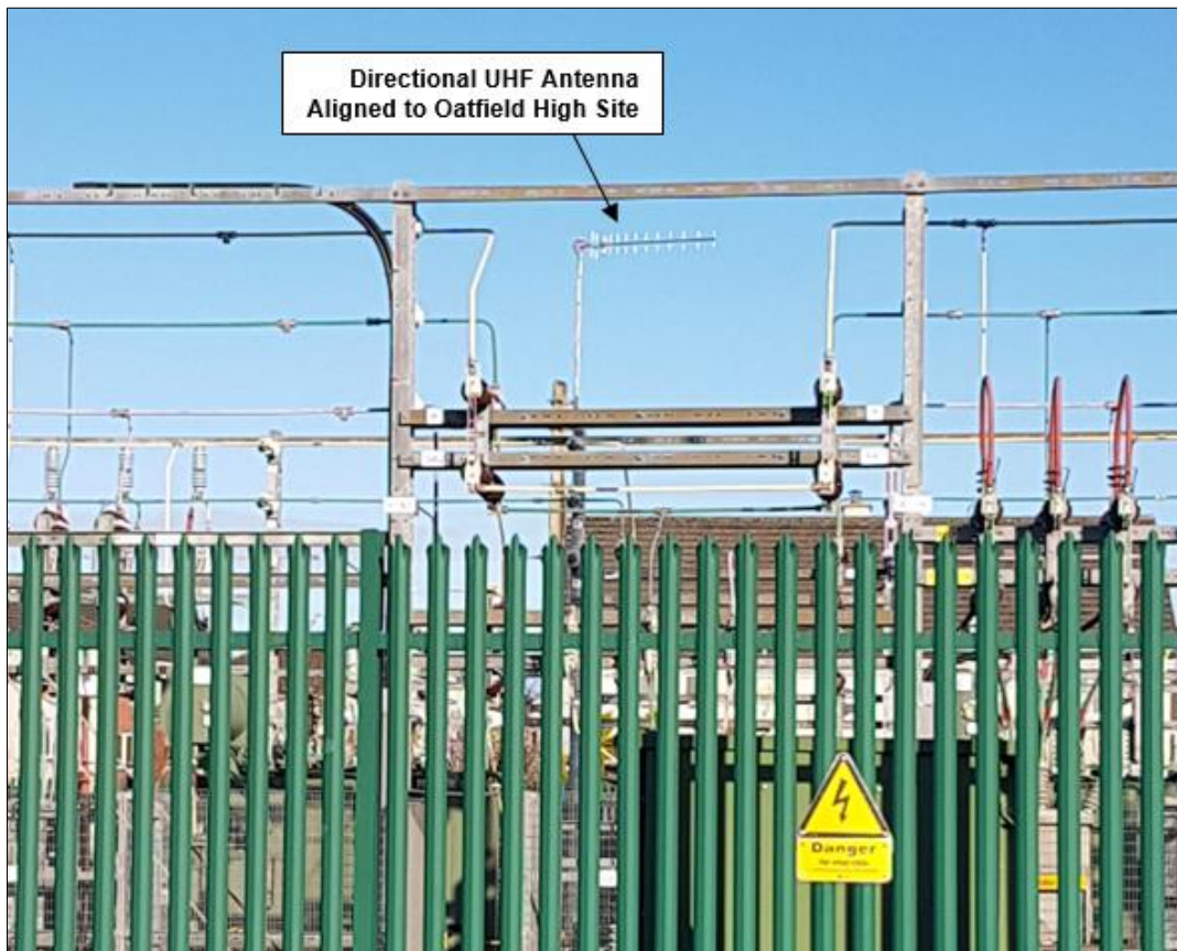
Figure 1. UHF Antenna at Ennis North 38 kV Site.
