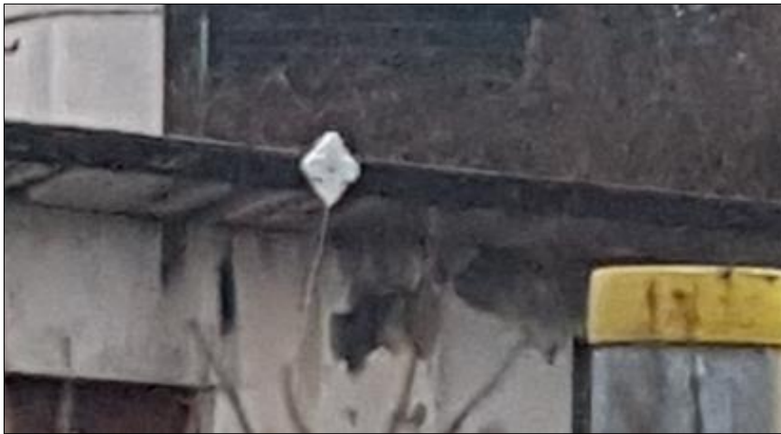
Figure 6. 3G/4G Broadband Antenna at Corrawarrin 38kV site.
