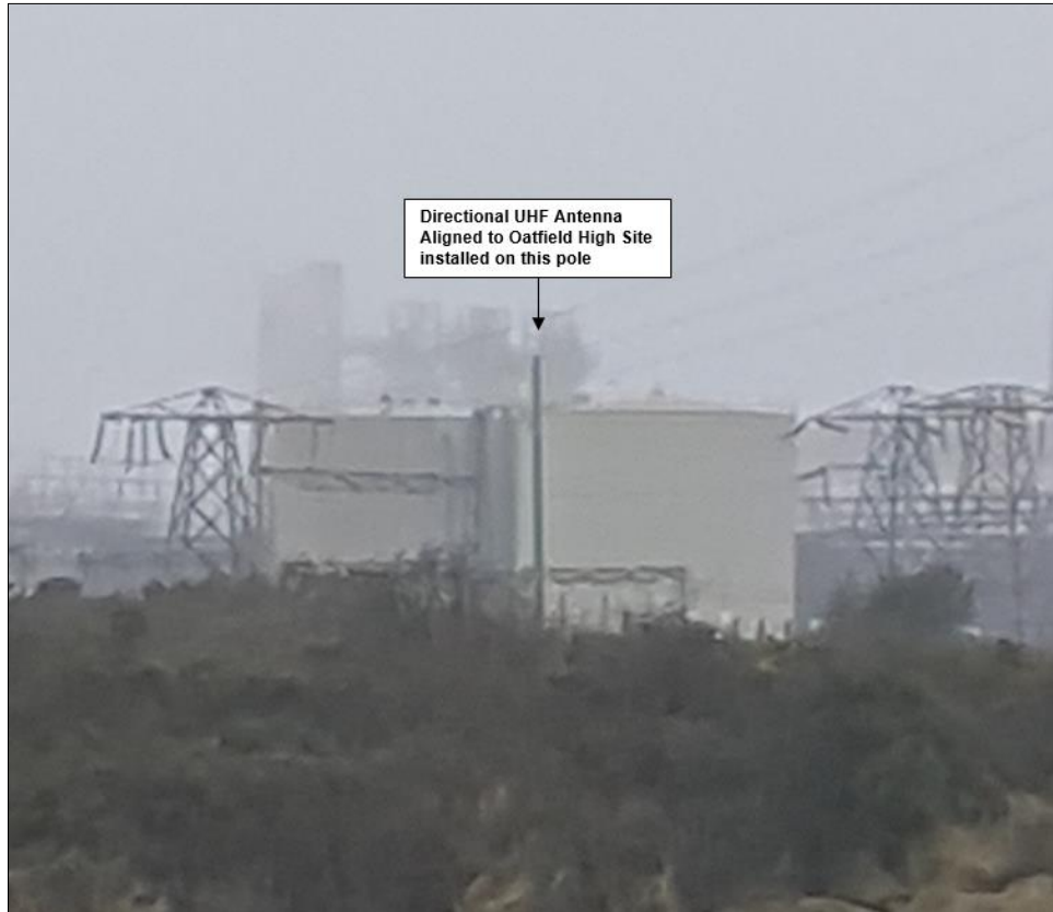
Figure 13. UHF Antenna at Aughinish 38 kV Site.
