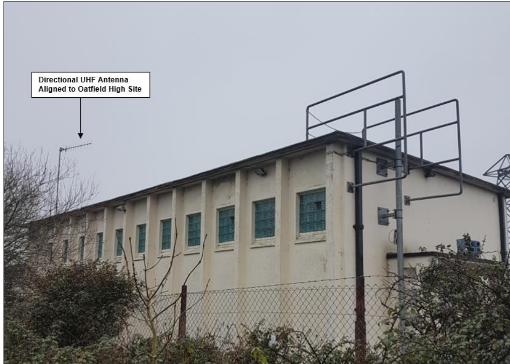
Figure 34. UHF Antenna at Rineanna 38 kV site.
