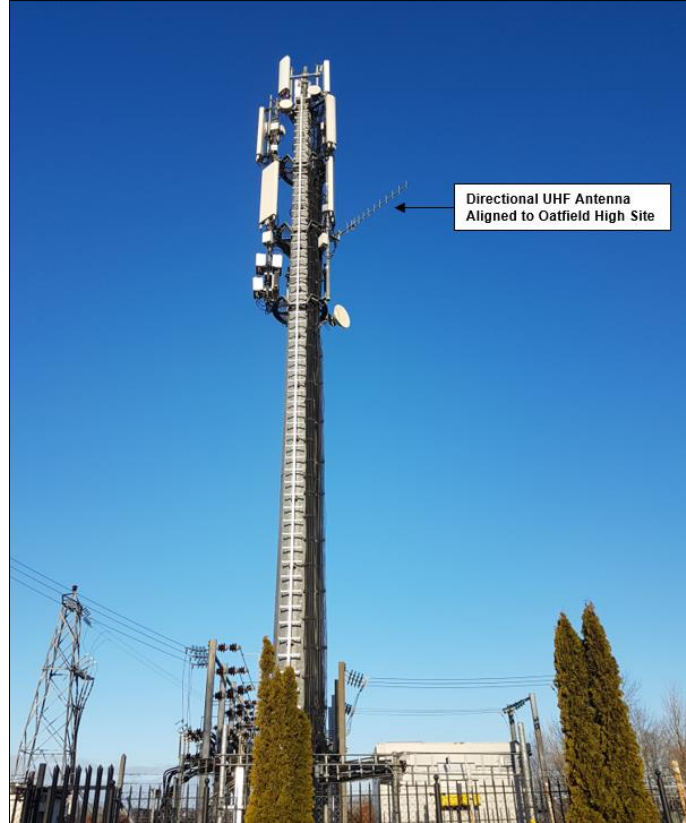
Figure 22. UHF antenna at Clarecastle 38 kV site.
