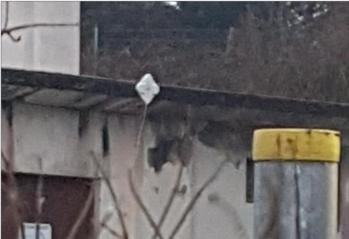
Figure 3. Example of a Cellular radio antenna at an ESB Substation
